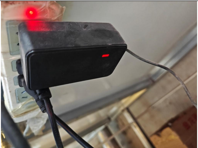
Battery charge check-8:15
